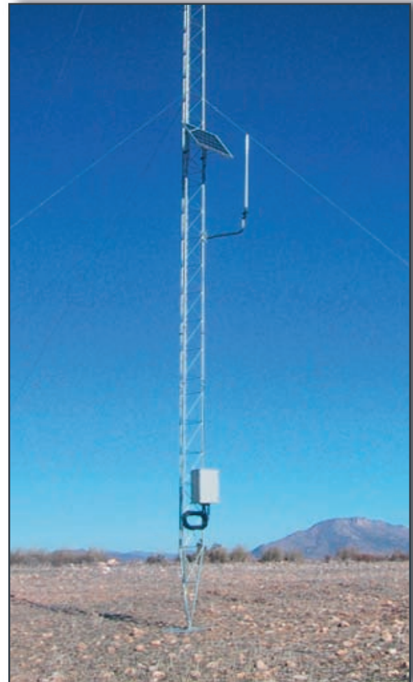
METEODATA-3000C Data Logger, a high gain GPRS transmitting antenna and a Solar Panel, mounted on the met tower
