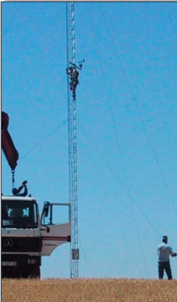
Mounting the wind sensors and the Data Logger / Transmitter, on a 60-meter stainless steel meteorological tower
